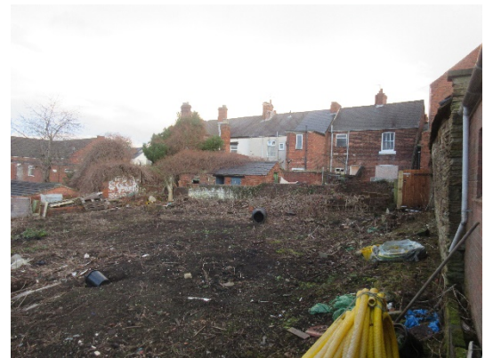
Photo taken from within site facing west towards the rear of buildings on High Street, showing site clearance
